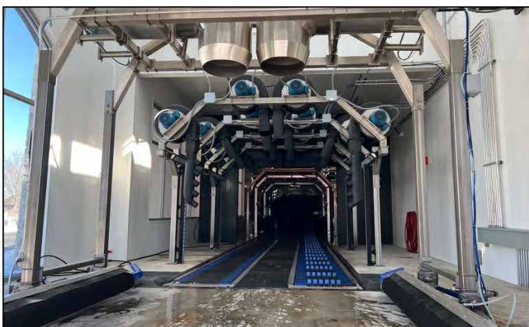
Figure 4 – Mount Prospect Car Wash Dryers
